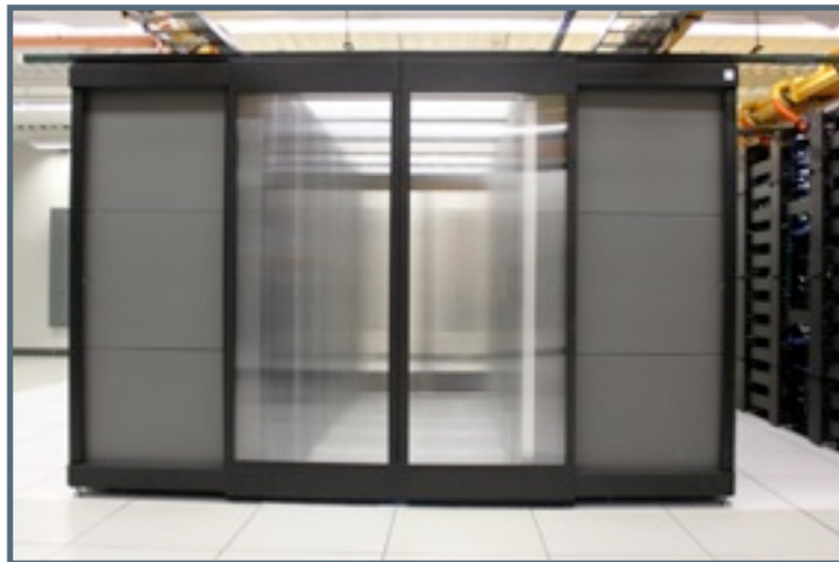
Cold Aisle Containment
